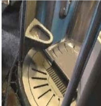
One set of Shower and Toilet in each HQ sleeping
